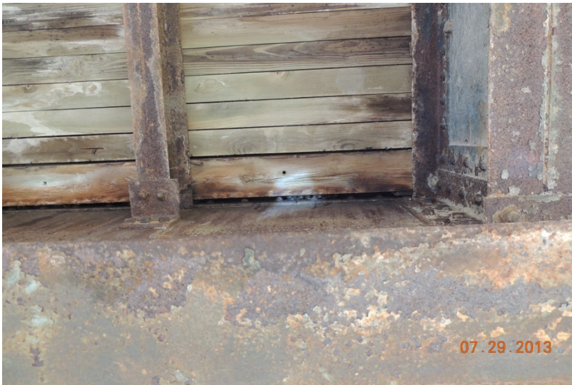
Photo 14: NLEBs Roosting Under a Timber Decked Bridge
